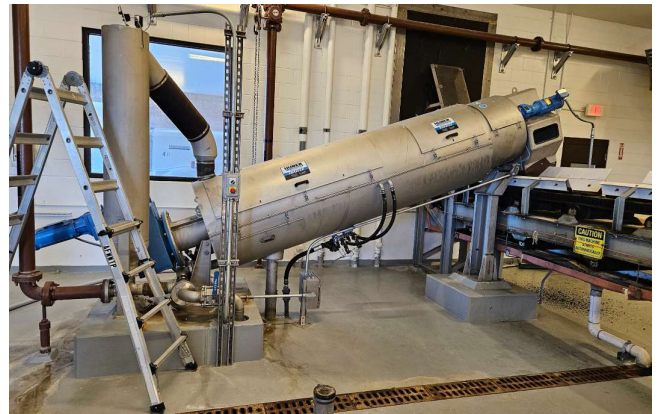
Photo 1: Example Screw Press for Solids Dewatering
