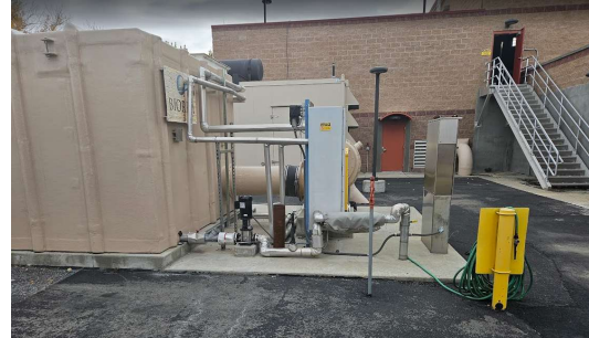
Figure 3: Treatment Plant Equipment
