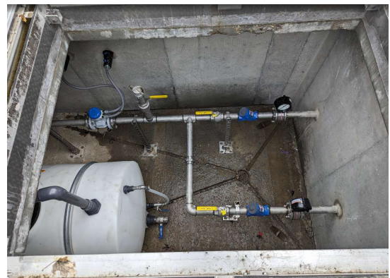
Figure 2: Typical lift station valve vault
